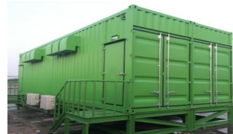
Terminal Electrical Equipment Containers
