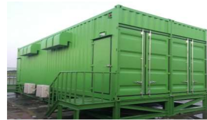
Terminal Electrical Equipment Containers
